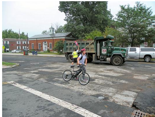
The repaving of Ridgewood Avenue added to the excitement of Back To School Day in Glen Ridge last Tuesday.
